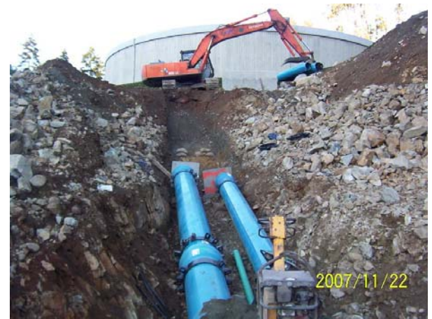
Inlet supply and outlet piping leading up to the reservoir site
