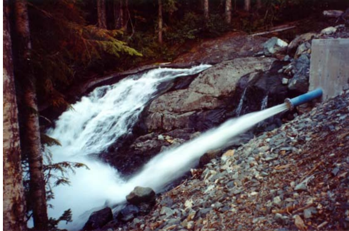
Discharge of 600 mm diameter siphon outlet into natural stream channel.
