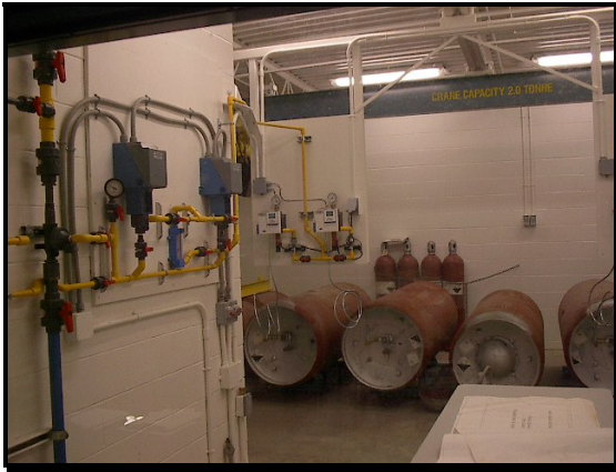
Chlorine Feed and Storage
