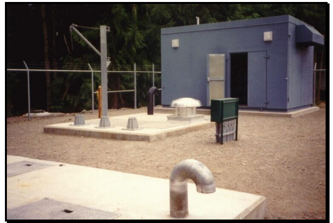
Completed station with valve chamber in the foreground, the wet well central, and the generator enclosed in background
