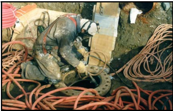
Preparing the pipe interior with abrasive blasting prior to the application of the coating material
