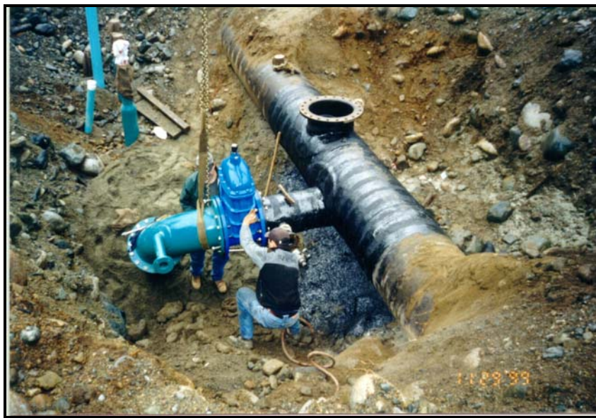
Installation of part of the 406 mm diameter inter-connection between the 750 mm and 1200 mm diameter water supply main.
