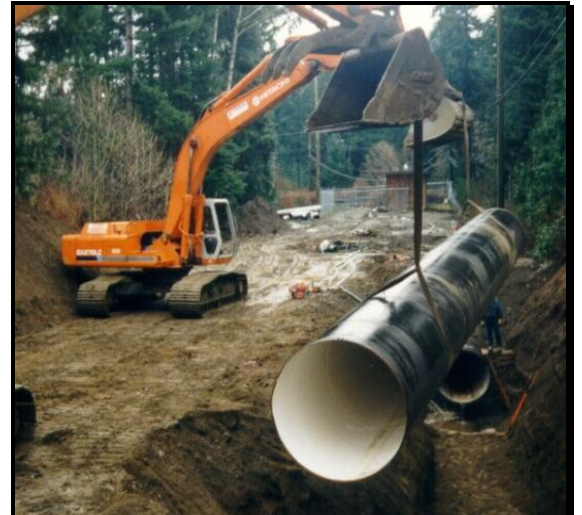
Lowering in the 1525 mm dia. chlorine contact pipe. This steel pipe provides additional contact time for the chlorine disinfection.
