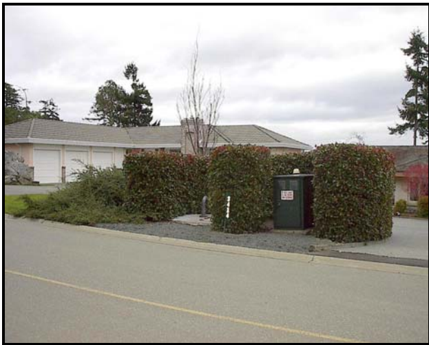
Pump Station Number 1 - Single Phase Underground Power Supply. (6 hp duplex pumps)
