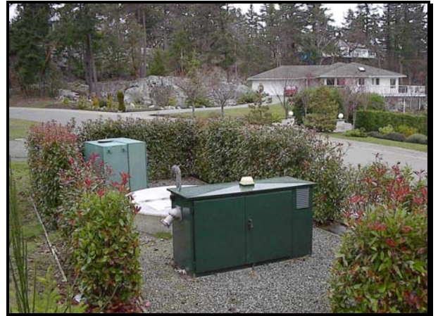
Pump Station Number 2 - Three Phase Underground Power Supply. (18 hp triplex pumps)
