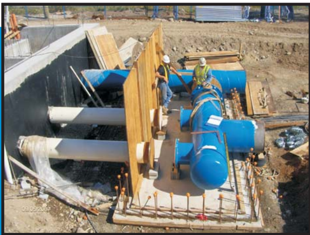
Suction and discharge headers in the south valve chamber
