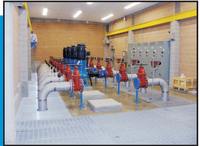
4 - 60 HP pumps and Motor Control Centre
