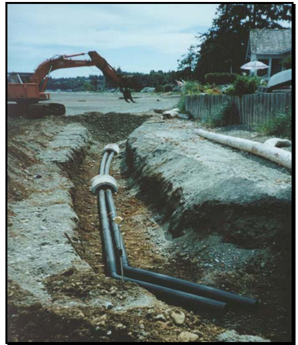
Twin force mains installed along the foreshore, with concrete weights to prevent flotation
