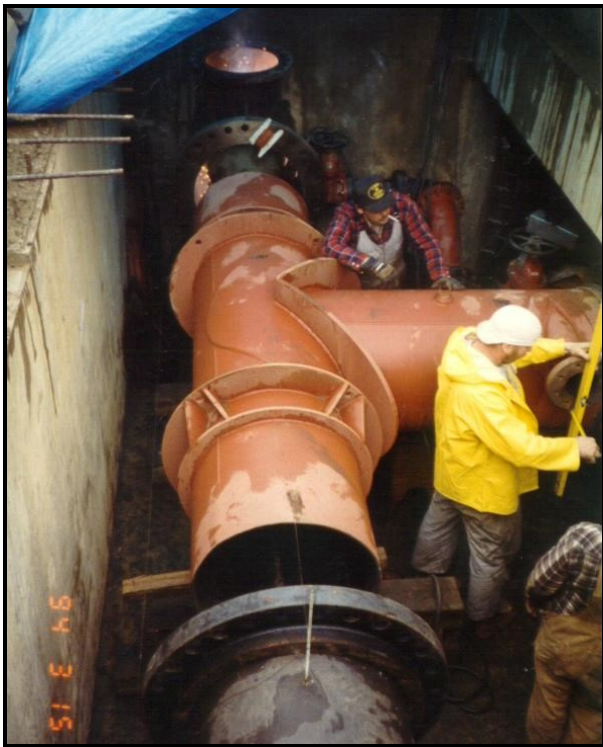
A 750x750x750 mm dia.. tee was cut into the existing 750 mm dia.. supply main to complete the cross connection between the two supply mains within the same chamber.
