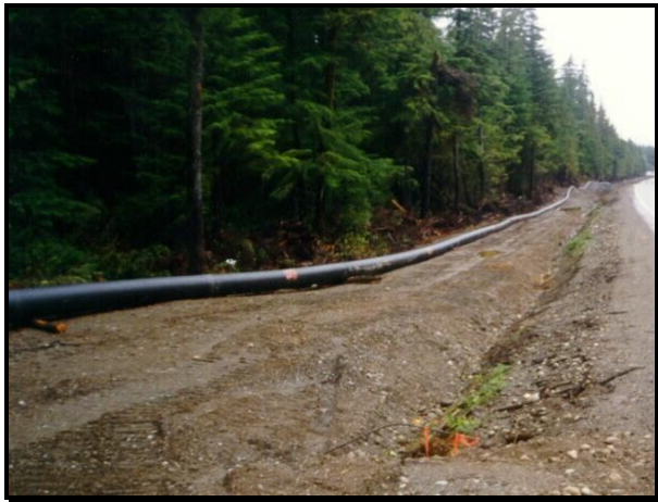
After fusion welding long sections, the pipe was strung along the right-of-way prior to trench excavation and installation.
