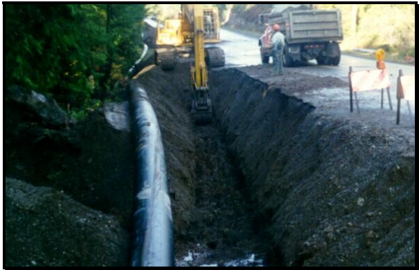
Pipe was lowered in after a long section of trench was excavated.
