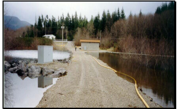
The well field under conditions of high ground water. An overflow to lower elevations controls the high water level.
